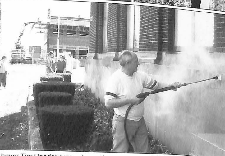
Above: Tim Reeder spray-cleans the outside library building. Right: It's looking great, as students clean-up in front of the Ferguson Center.
